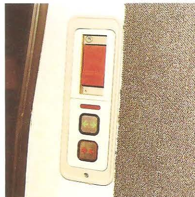
Local controls for passenger operation.
